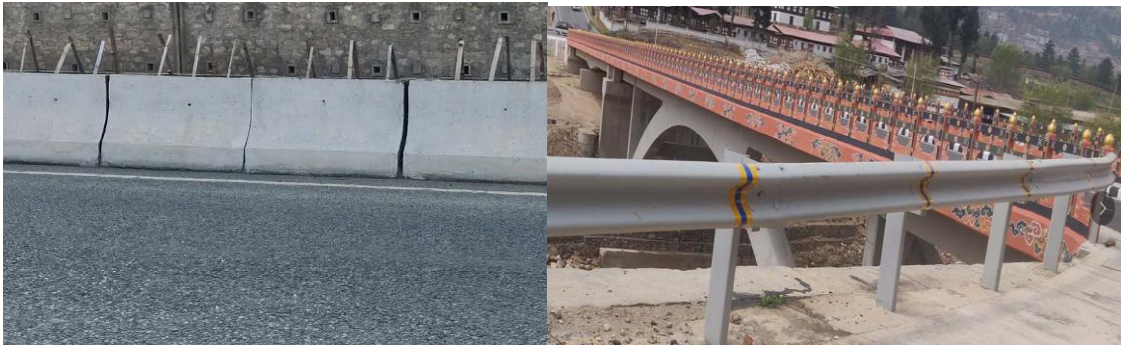
Fig: 3 a) Rigid concrete barriers, b) Semi-rigid W-Beam barrier on approach to bridge
